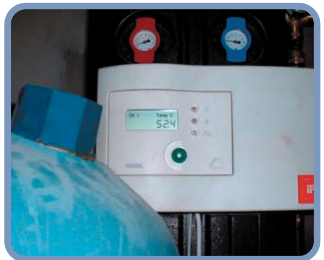
Figure 11: Control panel on the new solar systems
