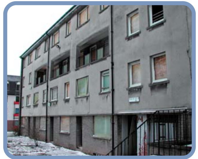
Figure 3: Flats before improvement
