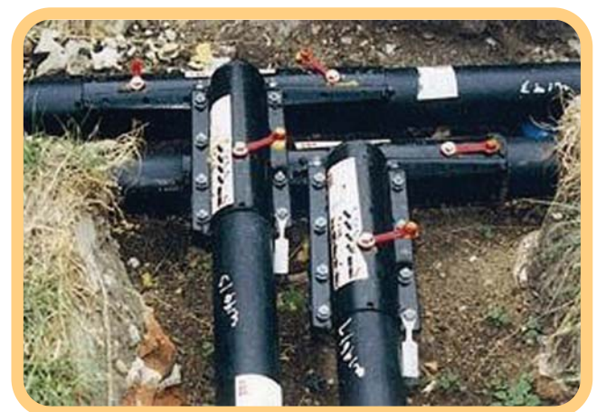
Figure 3: Pre-insulated heat mains
