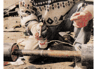
Connecting leak detection cables
