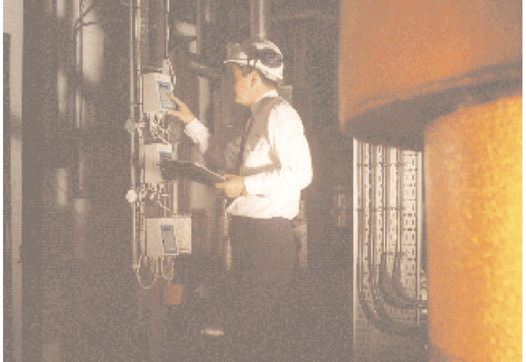
Figure 9 Good-quality maintenance can be achieved by selecting a contractor with a good understanding of CH systems
