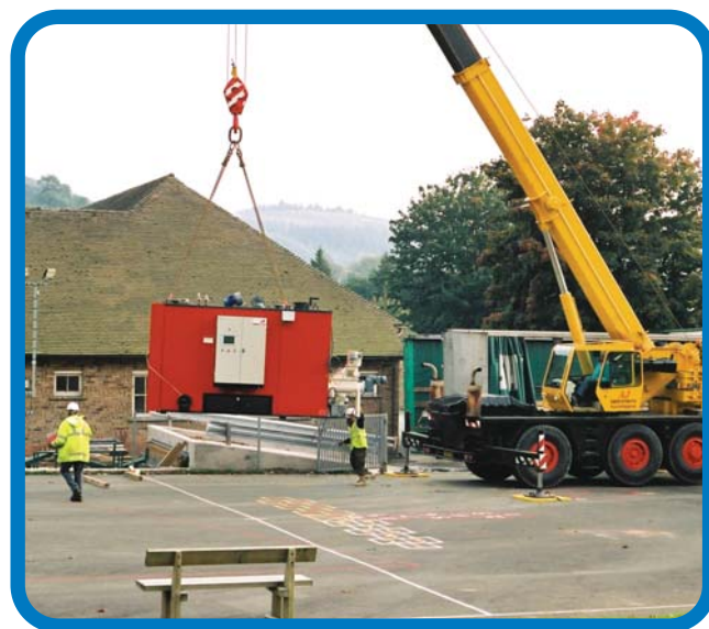
Figure 2: Arrival of boiler at Llanwddyn
