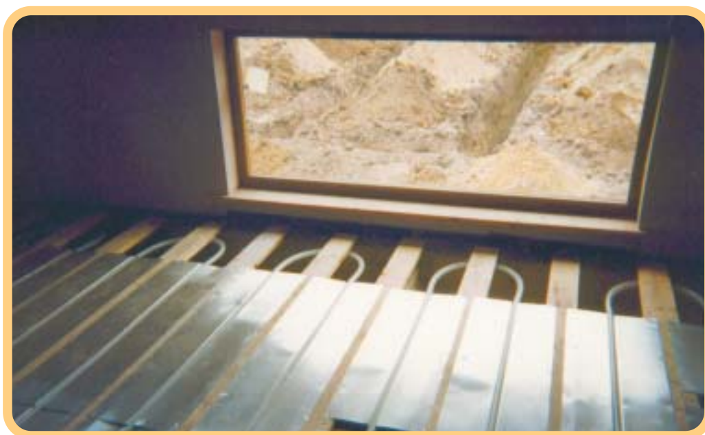
Underfloor heating system © R Rawlings 1997
