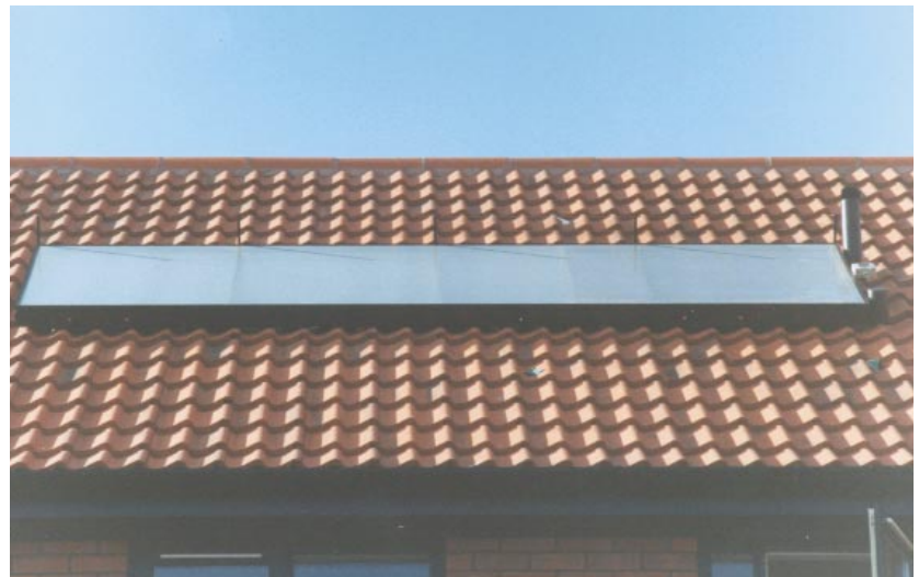
Figure 2 Close up of the installed selective surface flat plate solar collectors
