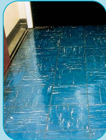
Asbestos-containing floor tiles
