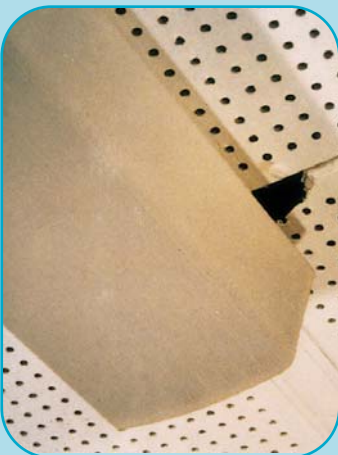
Perforated AIB ceiling tiles
