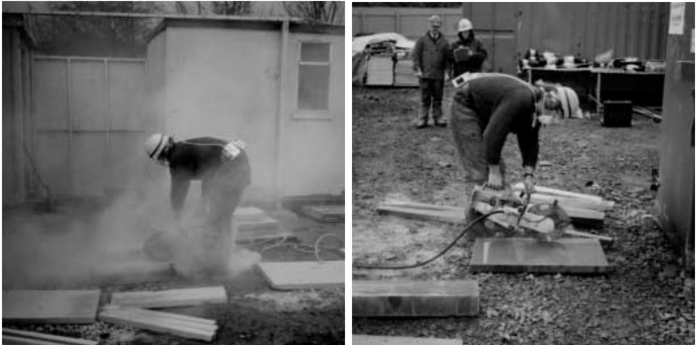
(a) (b) Figure 2 Slab cutting with mains supply water system: (a) without control; (b) with control
