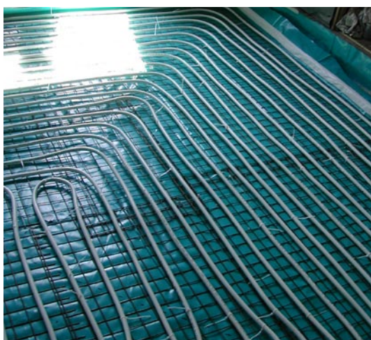
Figure 8 Underfloor heating system © J. Cantor
