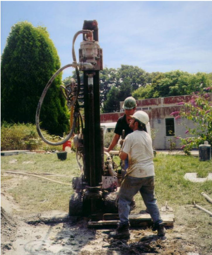
Figure 4 Typical drilling rig used for a vertical borehole based GSHP installation © R Curtis
